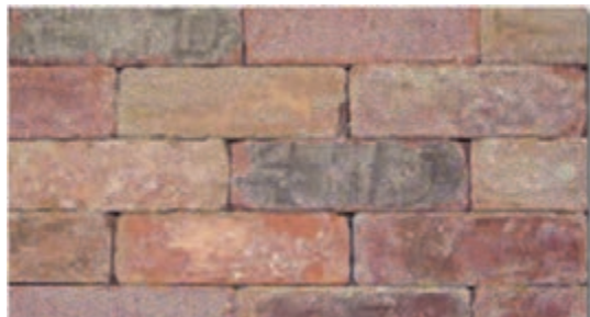
No Mortar Joint (Dry-Stacked)
